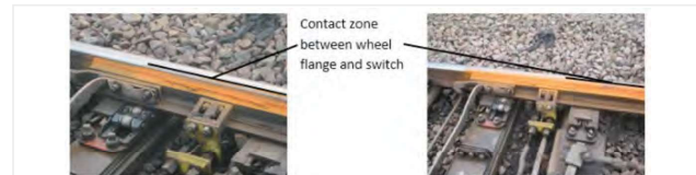
Figure 7: Left photo - untreated rail at WN572A at the switch toe. Right photo - both rails treated with the friction modifier at WN572A at the switch toe.
