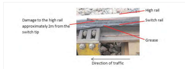
Figure 5: WN572A switch blade damage
